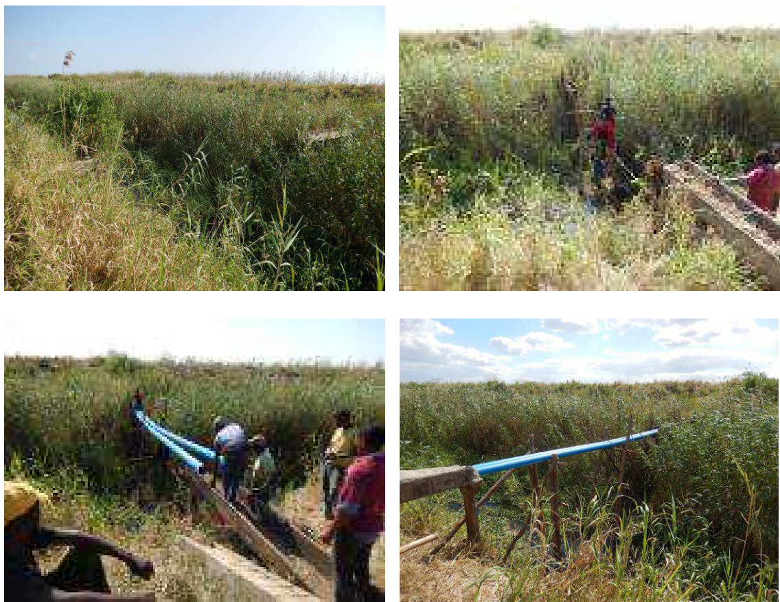
Photos 3.2: Replacement by PVC pipes for 2 spans (R12 in D11 area in 2013)
